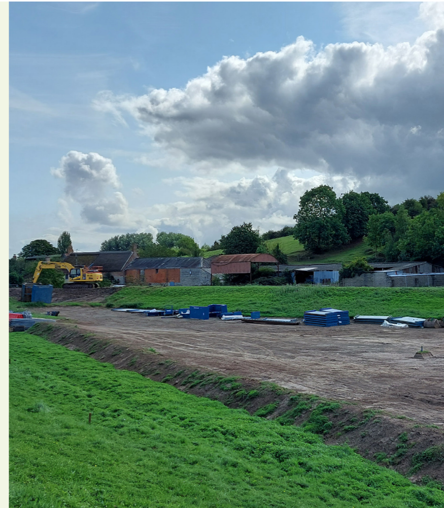
General view looking east of the work at Stan Moor cut off embankment
